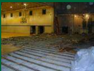
Removal of the stage in the old gym makes room for new classrooms.
